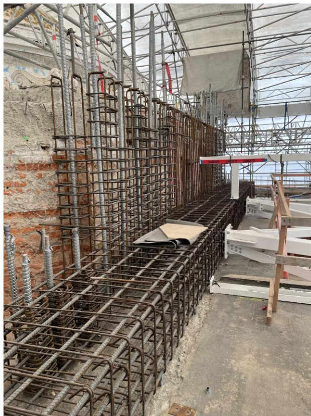
Figure 1.8 Reinforcing for concrete works around the dome and core roof with prestressing bars installed.
