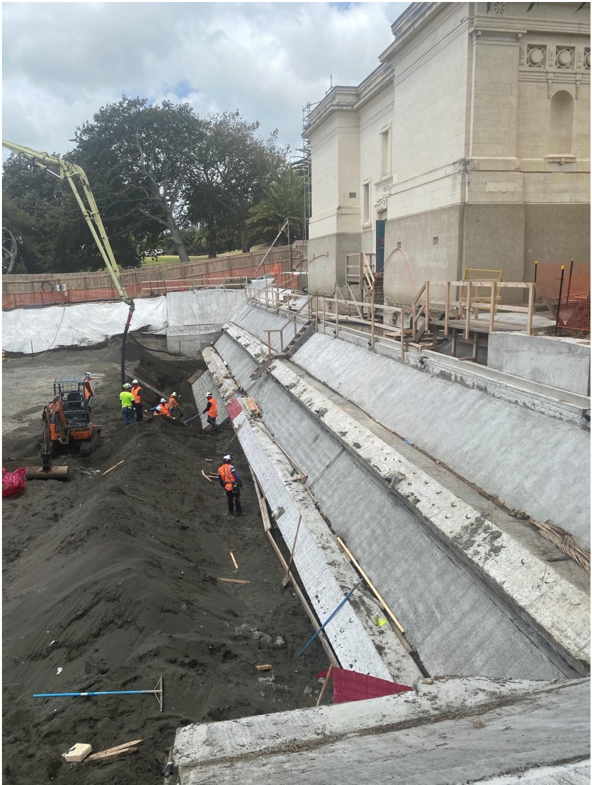
Figure 1.10 Temporary retaining wall at the north side of the original Sarjeant Gallery building nearly completed to accommodate the basement of the new extension building.
