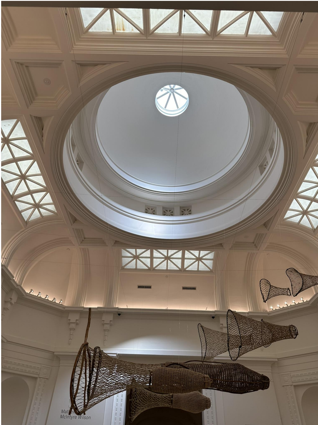
Figure 2.4 View of the dome roof and core area, with no structural interference inside.
