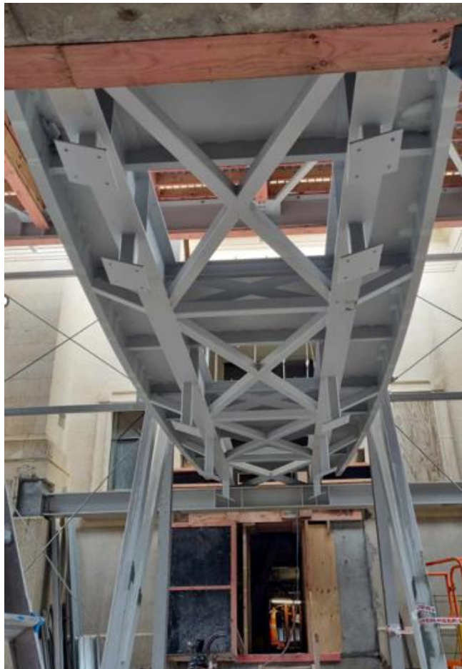
Figure 1.12 Bridge structure being installed amongst the temporary works at the north façade prior to being cladded in Maori carving.
