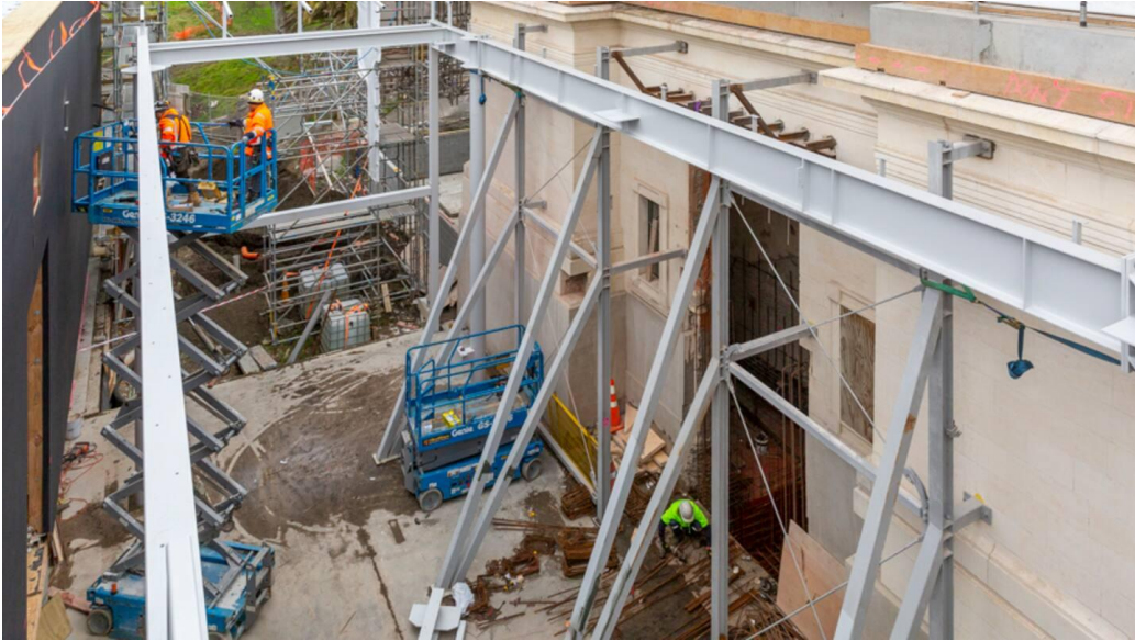
Figure 1.11 Temporary steel work to stabilise the north façade to allow relocation of the north entrance from the basement level to the gallery level and to allow a bridge structure to be installed. (Refer Figure 2 and Figure 1.10 for the original north entrance location)
