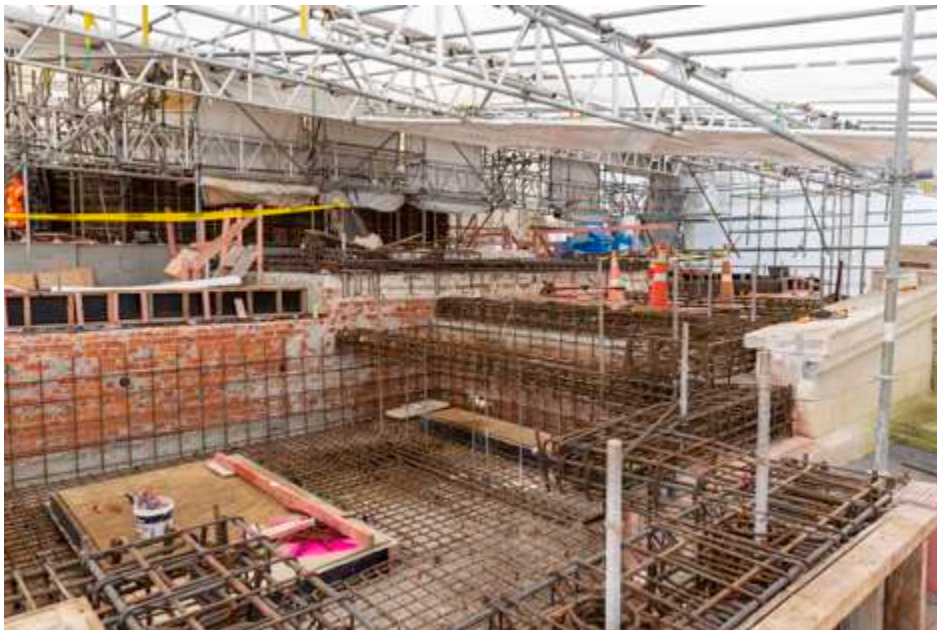
TOP: Ply being installed on the roof of Te Pātaka o Sir Te Atawhai Archie John Tairaroa BOTTOM: Complex steel frame works on the roof of the original Sarjeant Gallery building
