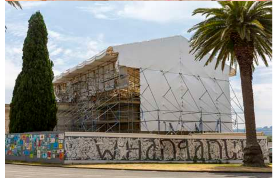
TOP: Demolition of old concrete and laying of drains is complete under the dome with newly completed suspended floors in the south wing visible in the distance
